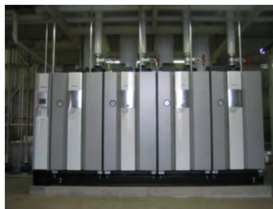
The boiler converted to LNG (liquefied natural gas) fuel
