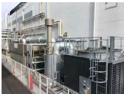
The cogeneration system
